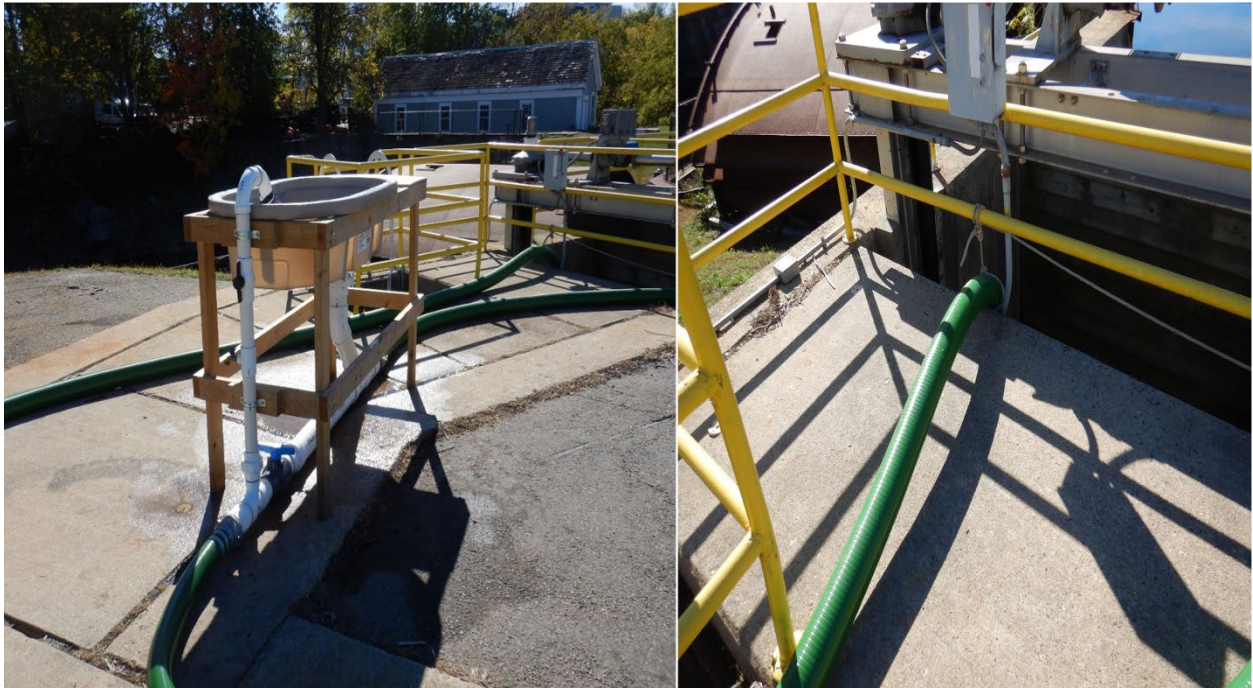
Figure 4-5. Fish injection system with 4-inch diameter hose connected (left image) and deployed at the fish bypass downstream of the forebay (right image)
